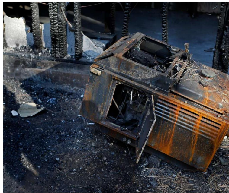
ency generator sparked a fire that burned the garage of his Grass Valley home during a PG&E power shut off in late September. Iacor / Special to the Chronicle
